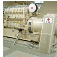
Power generator for emergency purposes
