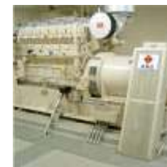
Power generator for emergency purposes
