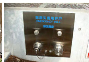
Drain (Emergency Wells)
