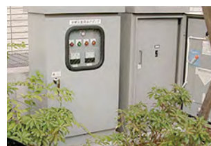
Operation System (Emergency Wells)
