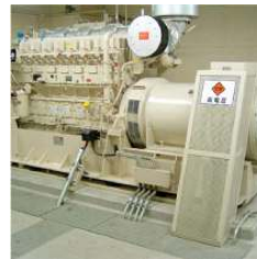
Power generator for emergency purposes
