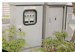
Operation System (Emergency Wells)
