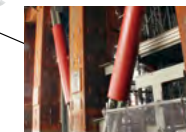
Unbonded braces (steel dampers) (82 installed in the building)
