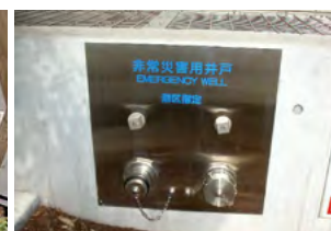
Drain (Emergency Wells)
