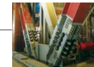
Brake dampers* (620 units installed)
