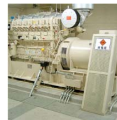
Emergency electrical generation system
