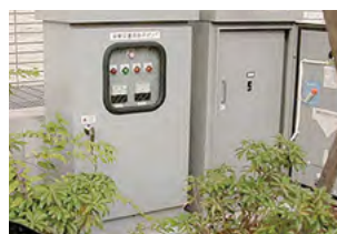
Operation System (Emergency Wells)
