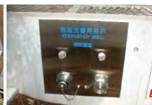
Drain (Emergency Wells)
