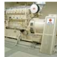
Power generator for emergency purposes
