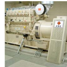
Power generator for emergency purposes
