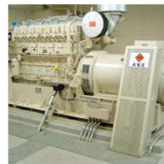
Power generator for emergency purposes
